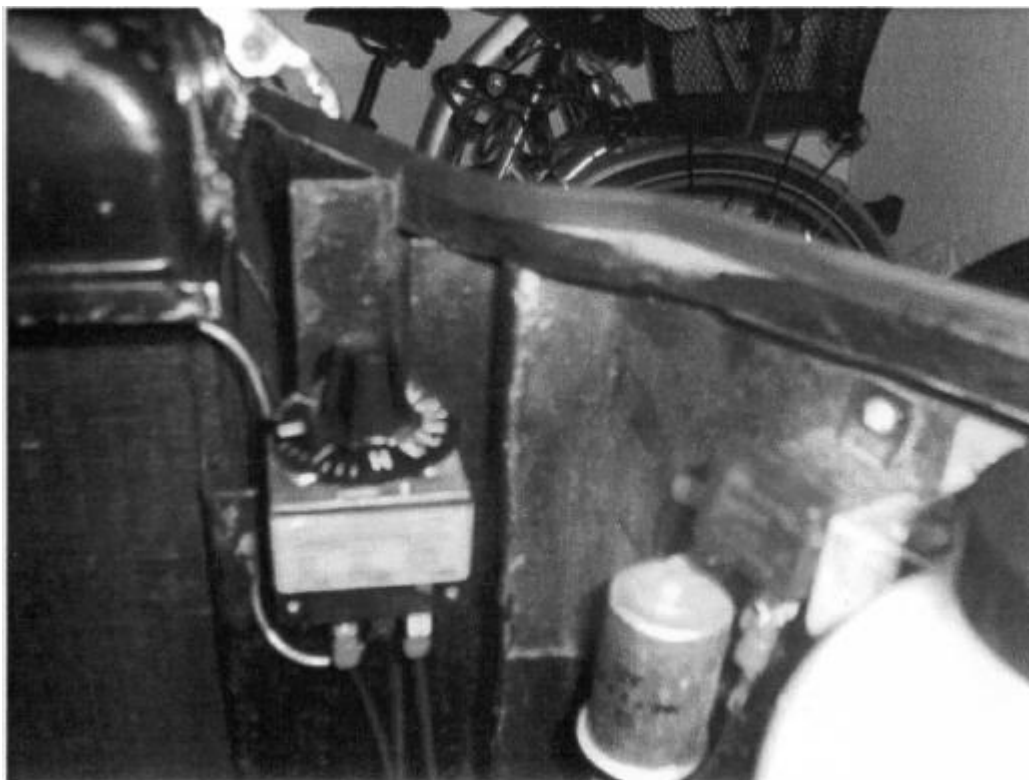
Another view of the pump
