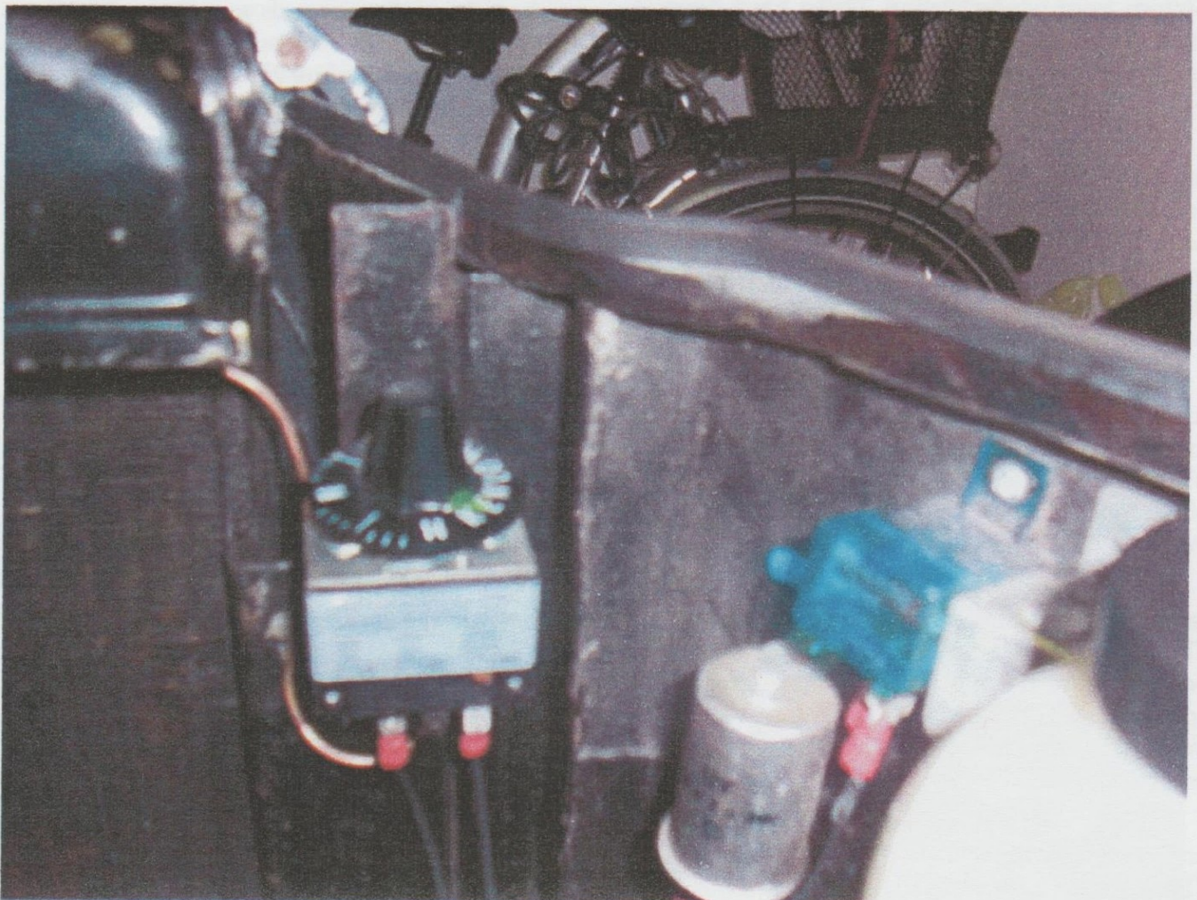
Another view of the pump
